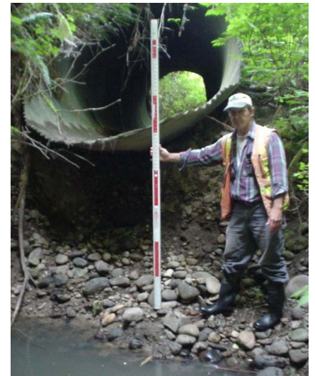
A pipe perched this high above the stream makes it impossible for salmon to migrate upstream.
