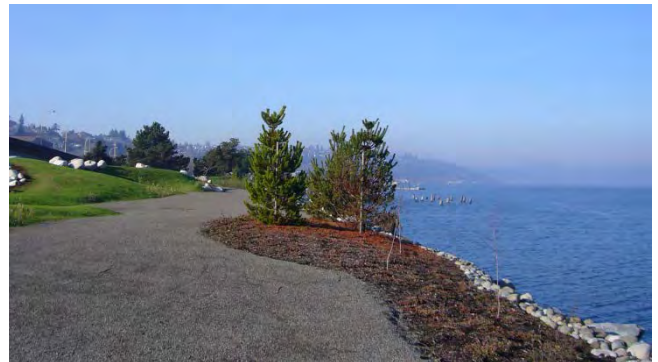
The City of Tacoma used a $455,000 ALEA grant to build a landscaped shoreline trail to the beach, restore the shoreline intertidal area to provide additional habitat, and construct an entrance gate to the Chinese Garden and Reconciliation Park on Commencement Bay.
